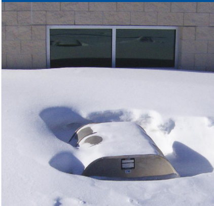
FIGURE 3 Rooftop hood in snow.
