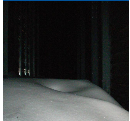
FIGURE 5 Snow in AHU.
